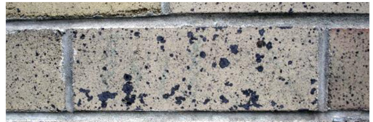
19. Spotted bricks, a pattern of dark spots on the surface of face brick caused by iron or manganese oxides. 38
