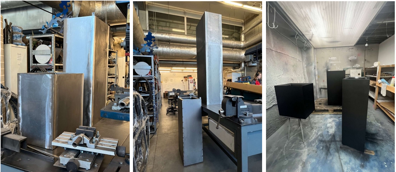
Figure 19 Construction of the full-scale monolith: welding the steel skeleton and panels at the Academy's metal studio (Wrocław, 2025). This stage marked the transition from prototype to final installation.
